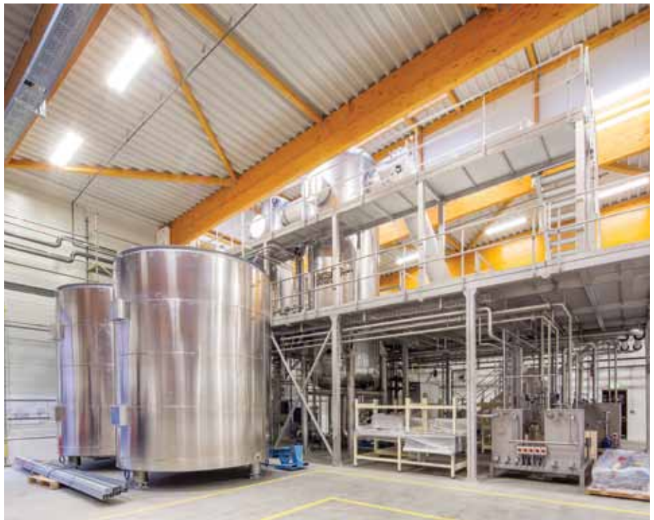
The new facility has three 25 tonne stainless steel tanks
